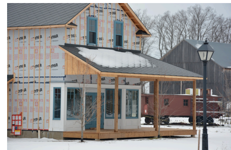
The general store at Moreston Village will soon be completed. The donation earlier this year from RTOERO Bruce/Grey Unit 1 is helping to make this project a success.
